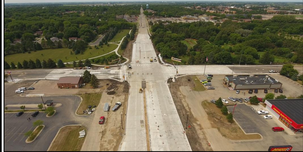
Project Photo: The completed intersection of 22 nd Ave. (just east of 22 nd Ave...looking west)
